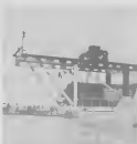
Two huge reactors arrived at Lago. The smaller 360-ton reactor is the Cu reactor of the Desulfurador. The larger 640-ton reactor is the Cu reactor of the Desulfurador. E reactor mas c pe
